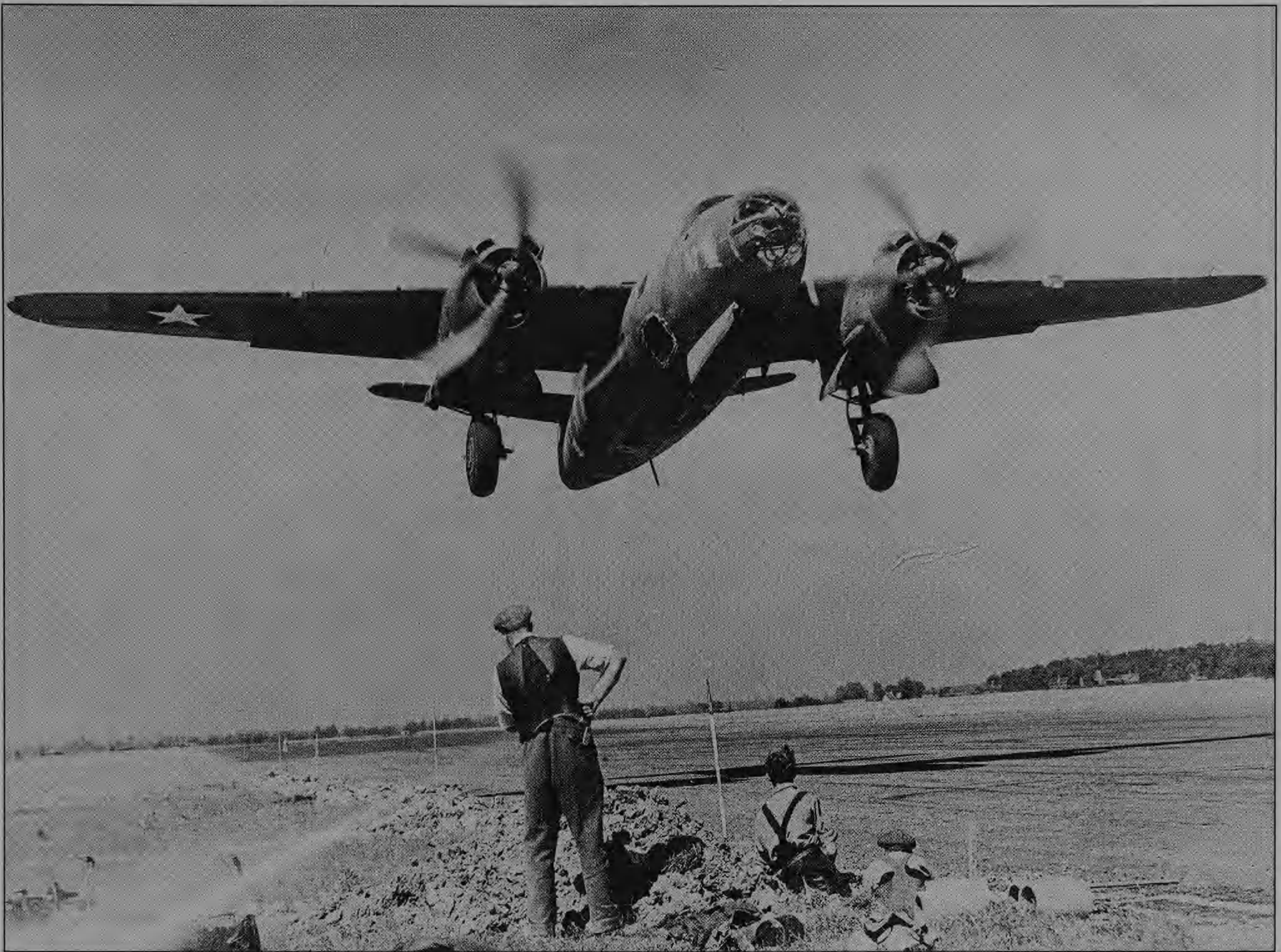
Seemingly unconcerned, British workmen at Great Dunmow, Essex, continue with runway construction as a B-26 Marauder of the 386th Bomb Group (Medium) lifts off. Note that the censor has obliterated the package guns on this photograph of this aircraft.
