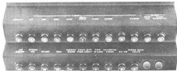
UPPER AND LOWER CIRCUIT BREAKER PANELS
