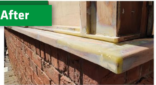
▲ Repair courtesy of DRM Carpentry DRY FLEX® 4 and DRY FLEX® SF used on application
