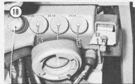
18 AUTO NAV (CHIN PACK) AIR AND PRE-HEAT SWITCH ACCESS (AFC 112 COMPLIANT WITH)
