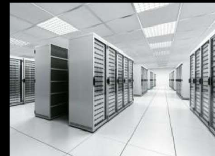
Typical DataCenter PUE > 1.4
