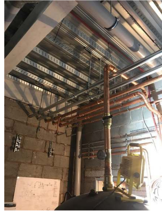
Dry risers and the heart of the building
