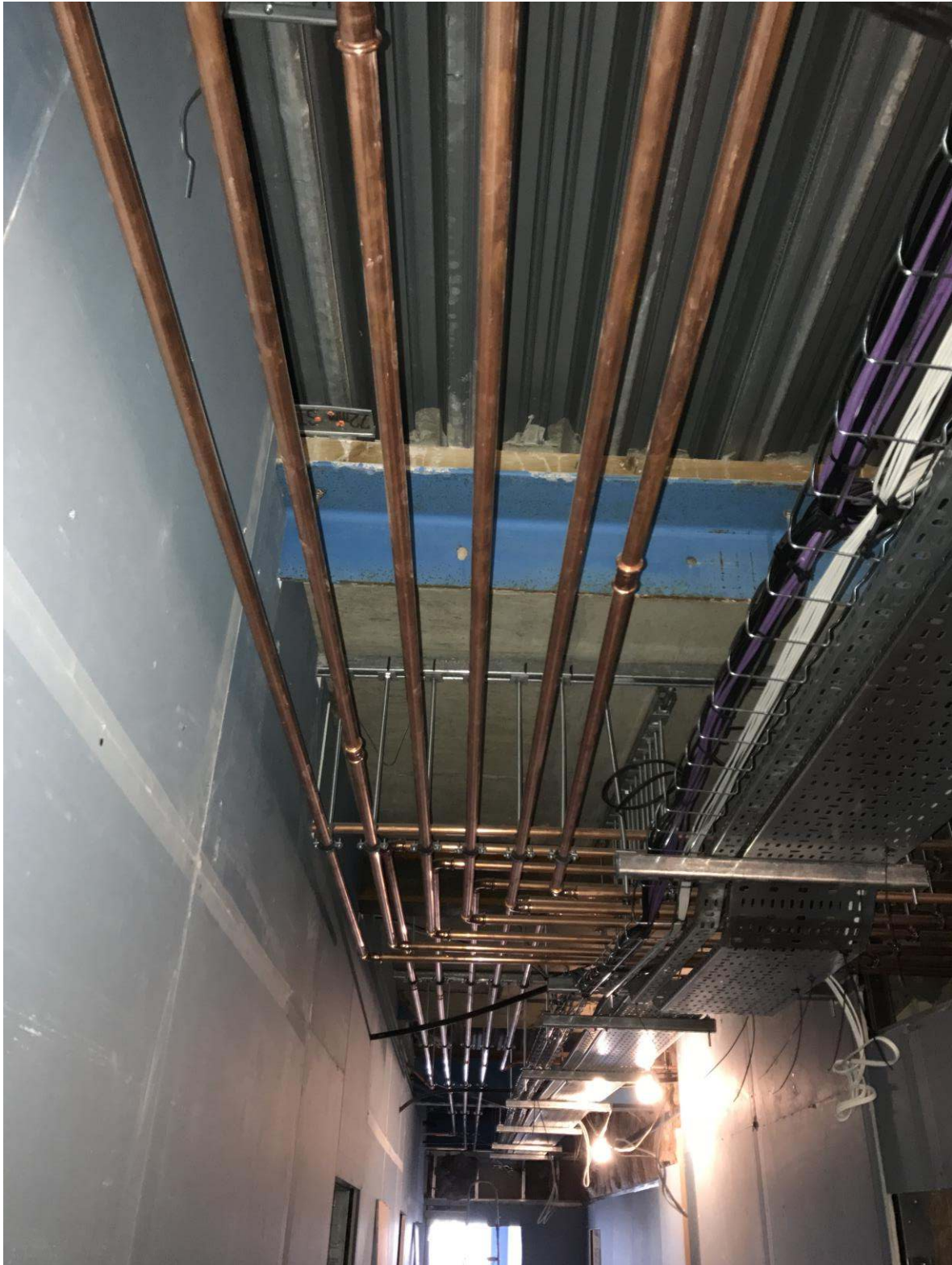
Fifth floor cold mains
