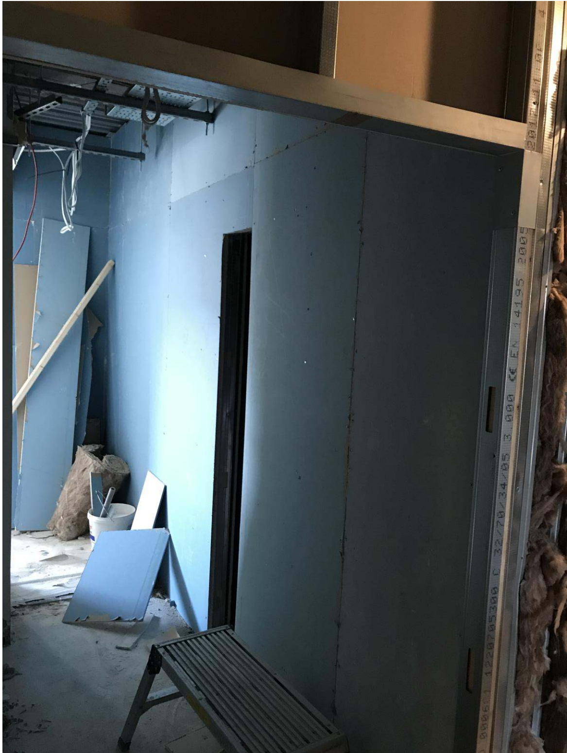
Fifth floor electric riser
