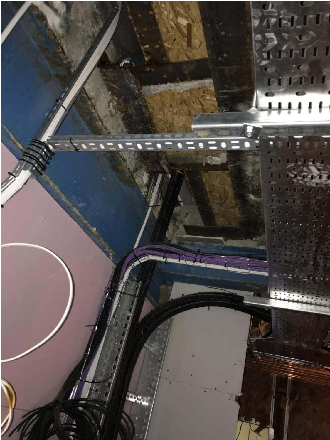
Fourth floor electrical riser
