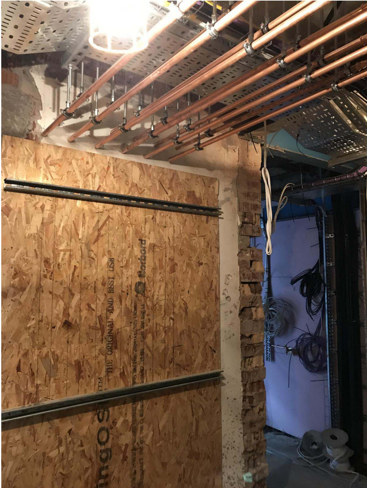
Fourth the floor cold water mains riser
