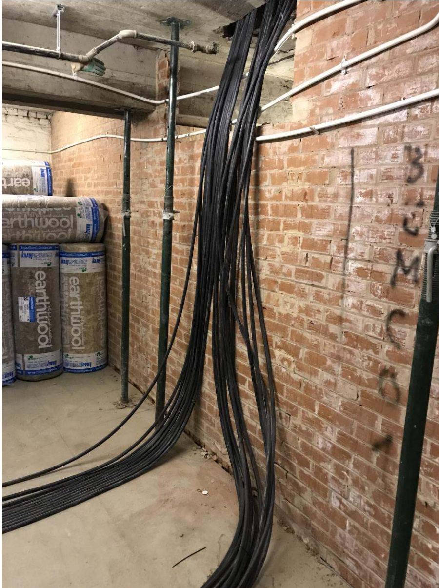
Lower ground, fifth and fourth floor apartment submains run to what will be meter room
