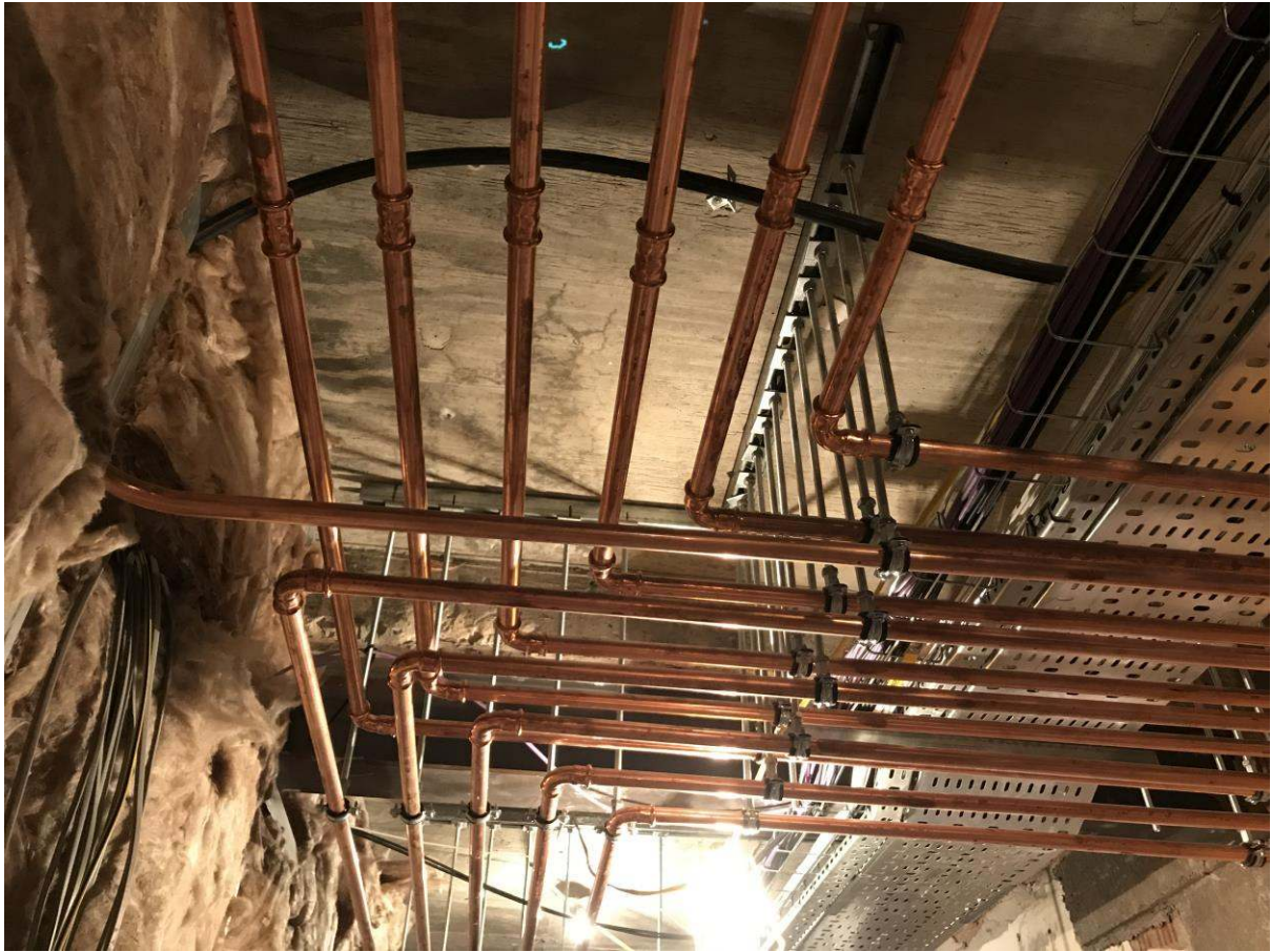
Fourth floor cold water mains
