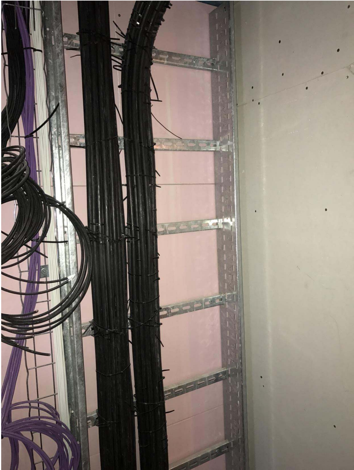
Fourth floor electrical riser-Apartment sub mains, TV coax, BT and door entry first fix
