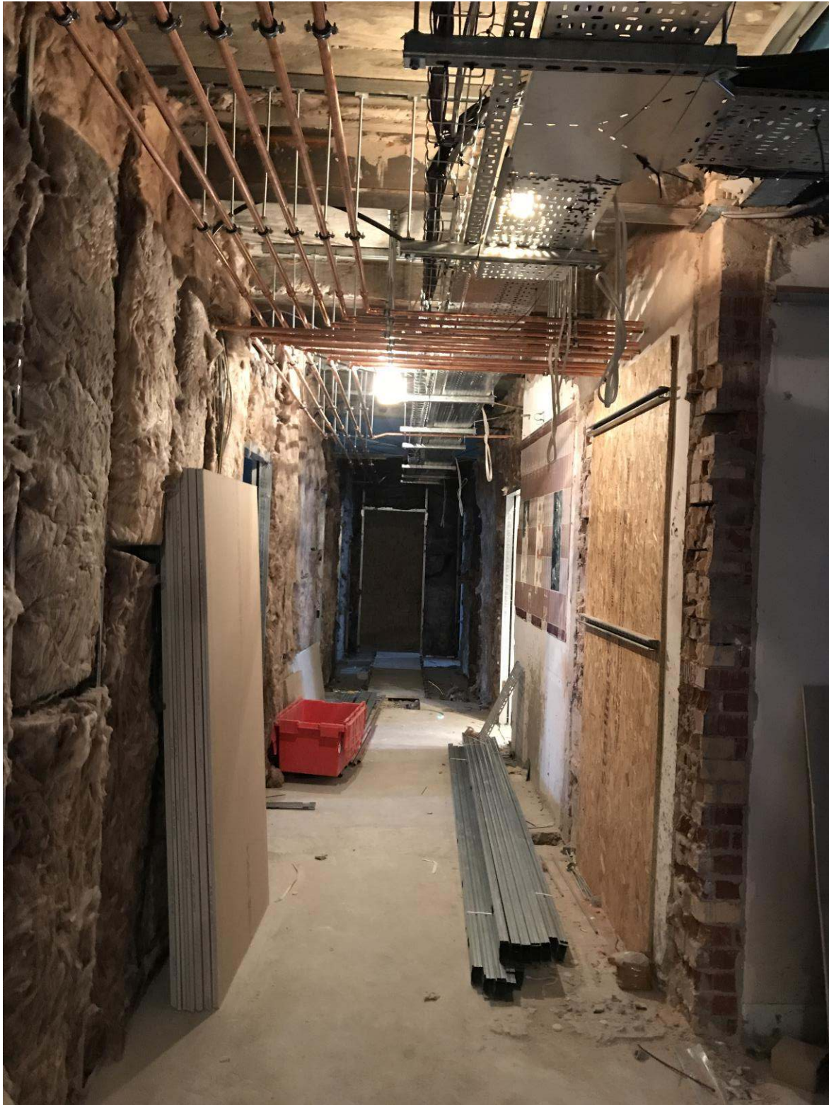
Fourth floor corridor, full M&E first fix, party wall insulation, ready for boarding
