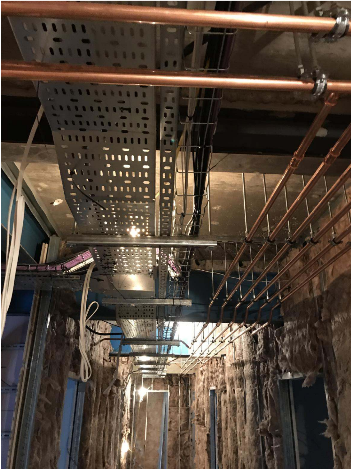
Fourth floor corridor, full M&E first fix, party wall insulation, ready for boarding
