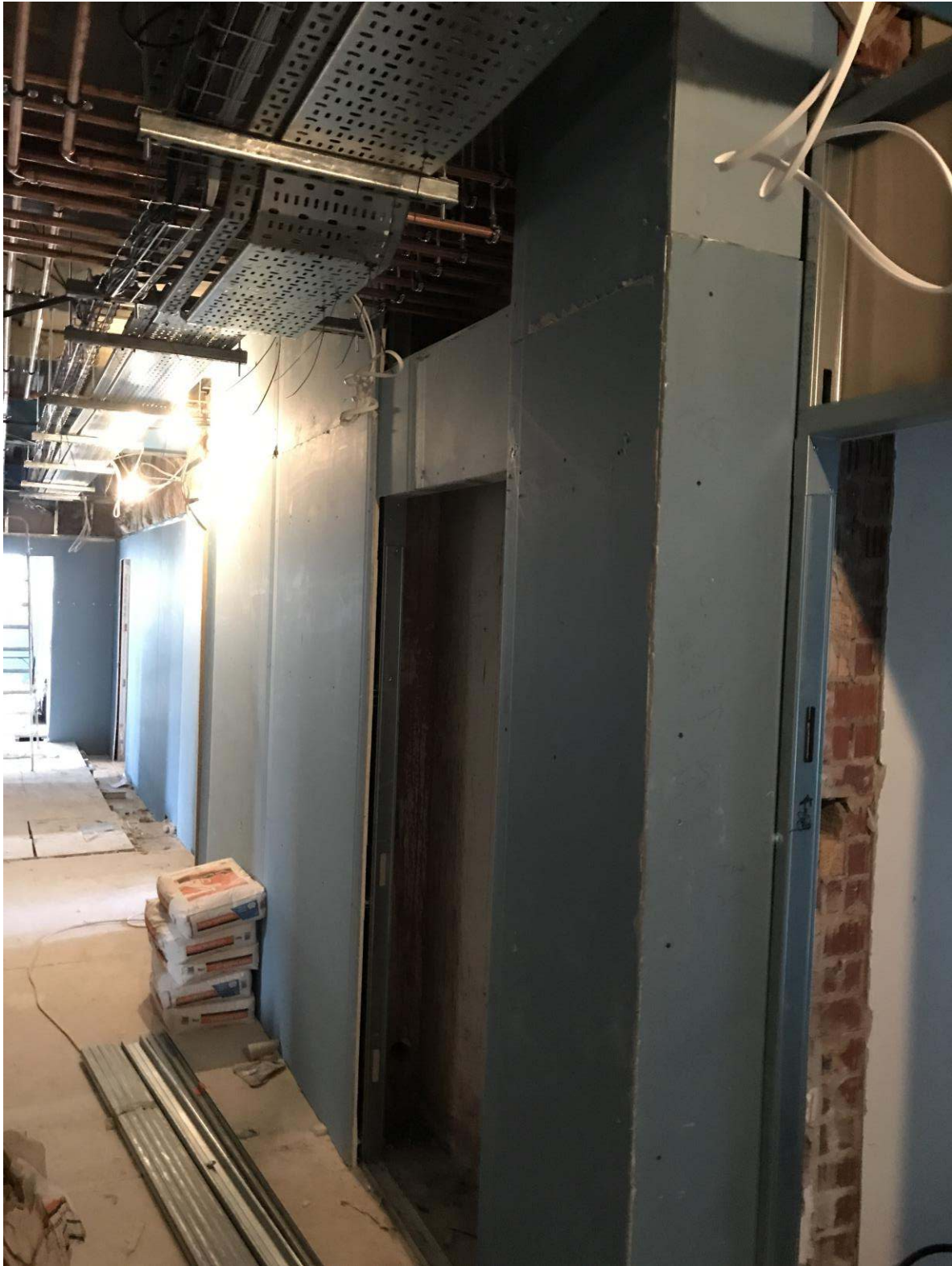
Fifth floor water riser
