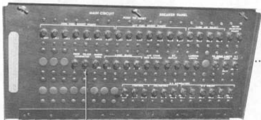
MAIN CIRCUIT BREAKER PANEL
