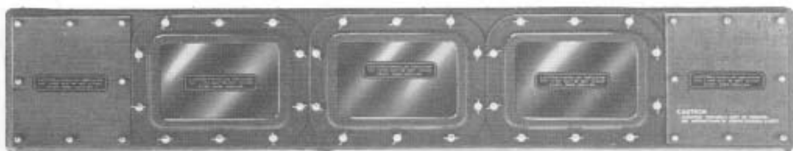
MAIN POWER PANEL
