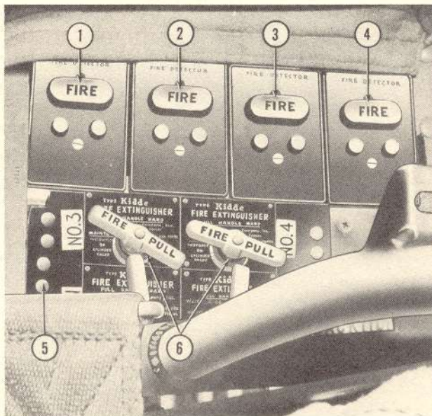
Figure 29 — Engine Fire Extinguisher Controls
