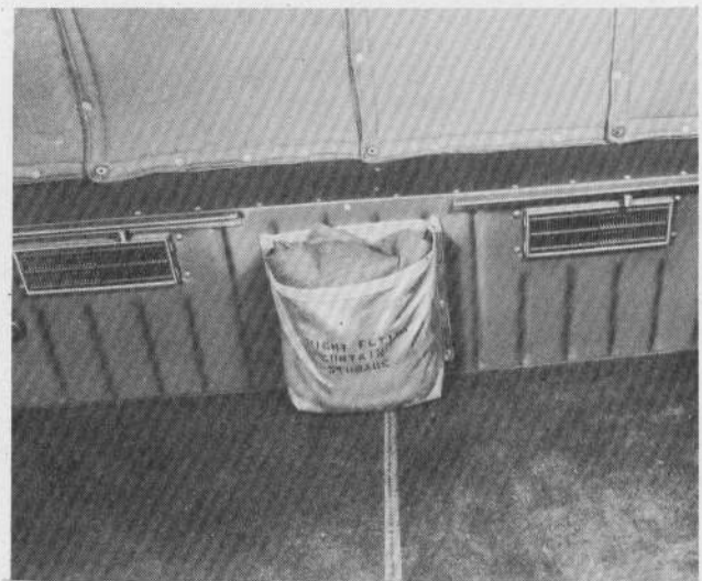
Figure 60—Heat Registers in Radio Compartment (B-24J)
