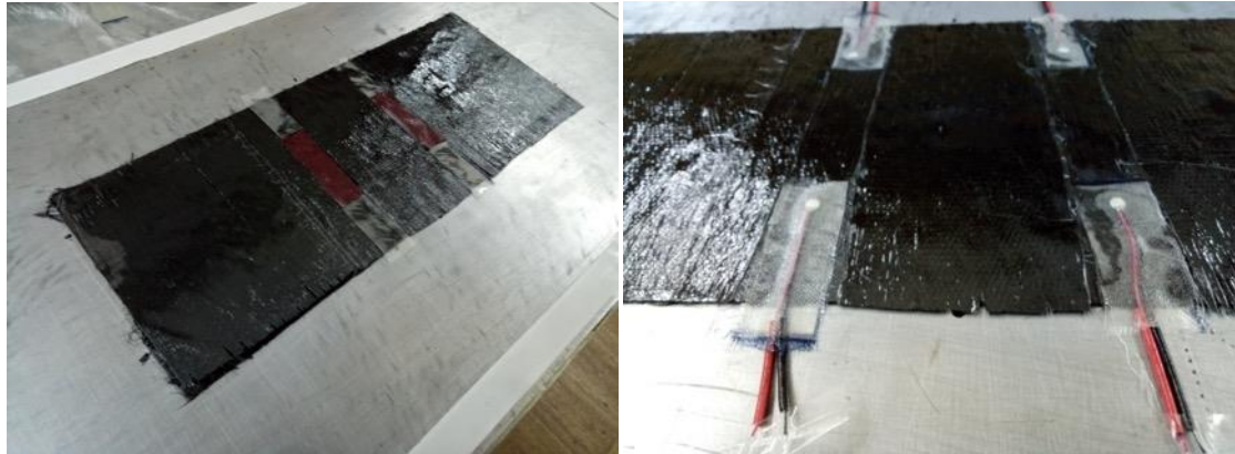
Figure 80. Installation of the sensors with removal of reinforcing material from the area of sensors installation
