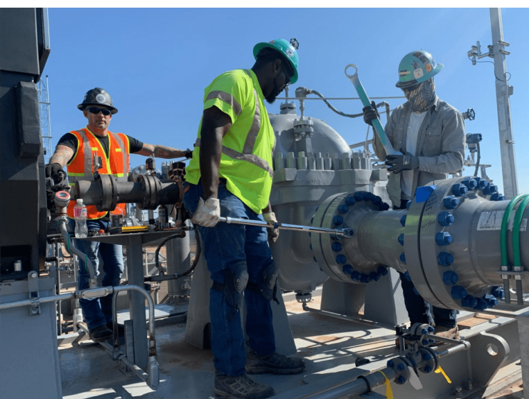
Tightening flange bolts as the laser shaft alignment system measures any shaft deflection.
