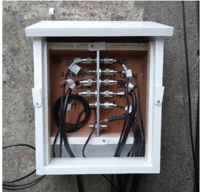
Fig 11 Box in place with cables from the house connected to the antenna coax cables
