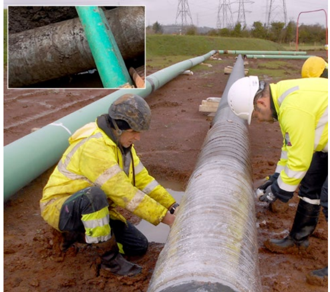
Denso™ Clear Outerwrap is applied whilst the ARO is curing, then removed once fully cured. The undamaged Denso Bore-Wrap™ is visible after the pipe is pulled (inset).
