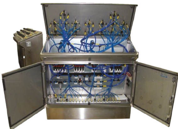
Water Treatment Controls for a UK Nuclear Power Station
