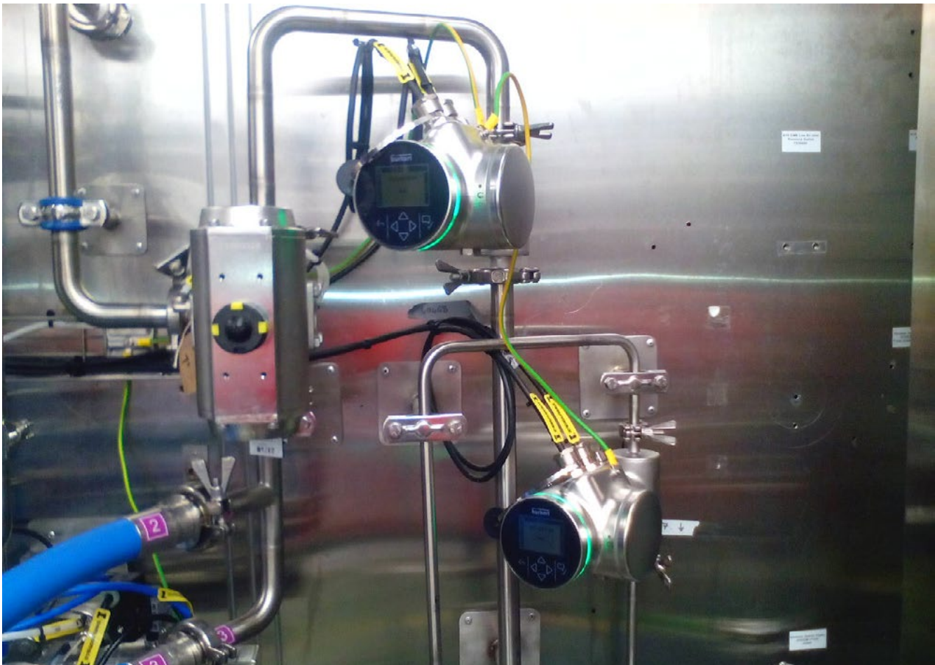
The FLOWave offers a very compact footprint, a key priority in this project
