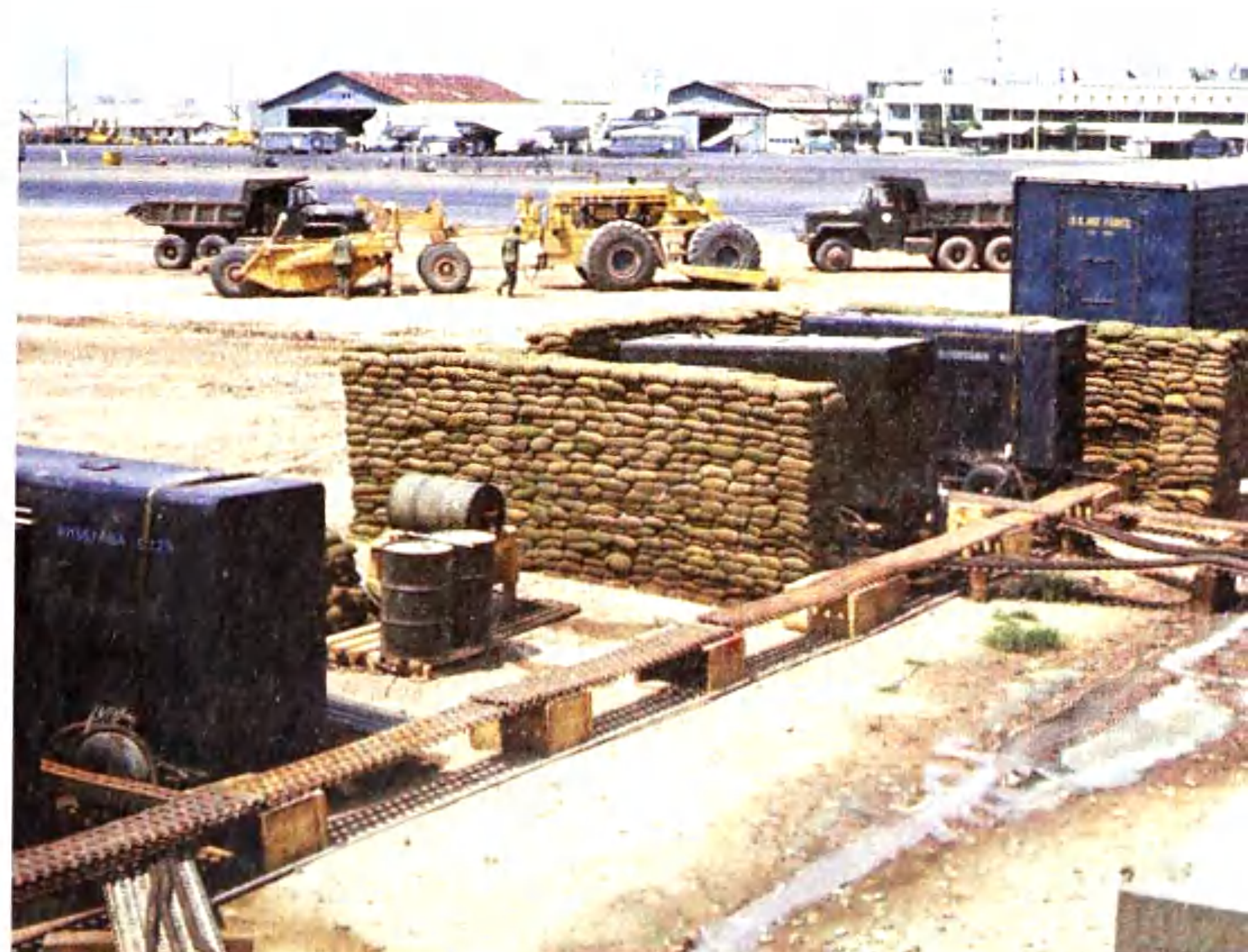
Special Protection. The PPIF's crucial electrical generators were given additional protection. Jim Ifland
