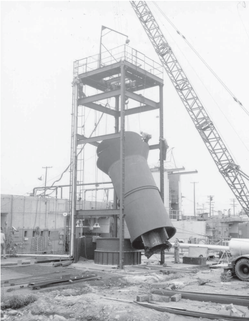
Figure 3.5. Construction of the 1/6th-scale silo model. Note the two workers at the center of the photo. The launch duct and exhaust duct were installed in one piece, and transportation through the streets of Los Angeles was quite an event. Courtesy of Rollo Pickford.
