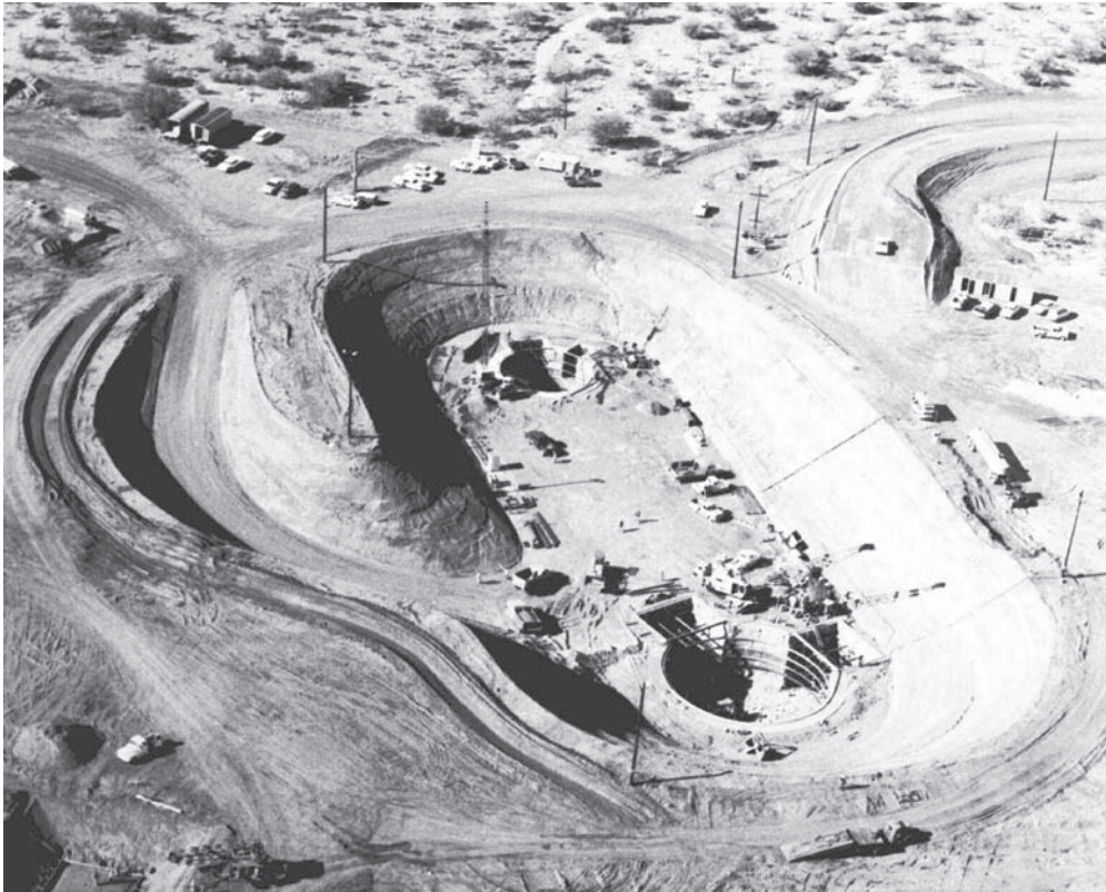
Figure 5.6. Excavation of both the launch control center and the silo shafts is well underway at this site of the 390th SMW, Davis-Monthan AFB. The large rectangular vaults on the side of the silo shaft are for the air intake and exhaust shock delay tubes. The electromagnetic shielding was welded to the ring beams visible at the top of the partially excavated silo shaft. Courtesy of the Titan Missile Museum National Historic Landmark Archives, Sahuarita, Arizona.
