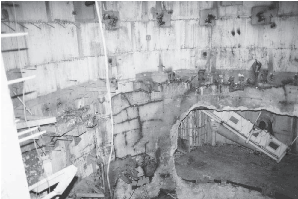
Figure 10.2. The diesel generators were recovered from Level 3 of the silo by using plastic explosives to open the 1.5-foot-thick launch duct wall clad with 0.5-inch-thick steel plate. This photo shows the results of the recovery effort at one of the abandoned Titan II launch complexes at Vandenberg AFB, California. Courtesy of Fred Epler.
