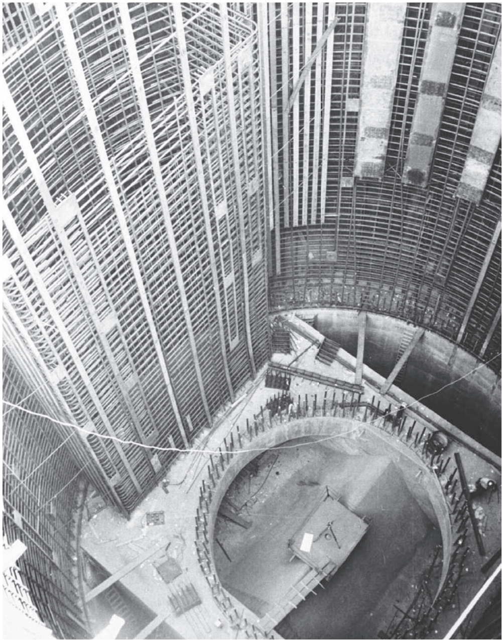
Figure 5.7. The silo is ready for the slipform concrete pour. The ring of rebar at the bottom of the silo is the connection for the launch duct structure. The completed flame deflector is clearly visible. The large vertical steel strips are anchors for the 100,000-gallon hardened water tank structure. Courtesy of the Titan Missile Museum National Historic Landmark Archives, Sahuarita, Arizona.
