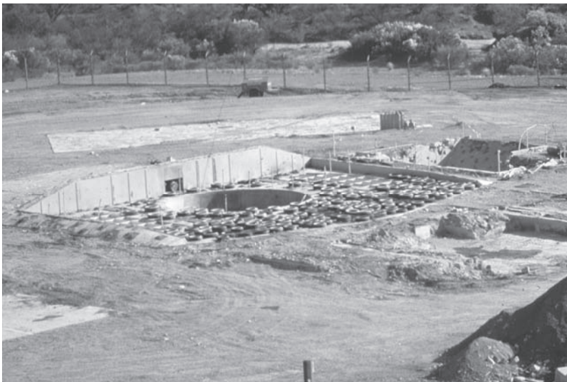
Figure 10.4. Launch Complex 570-8, 390th SMW. The silo closure door has been dismantled, the cooling towers have been removed, and the site is now ready for the demolition of the headworks. Rubber tires were lashed together and placed on the surface of the area to be demolished in an attempt to contain the debris. Courtesy of the Titan Missile Museum National Historic Landmark Archives, Sahuarita, Arizona.
