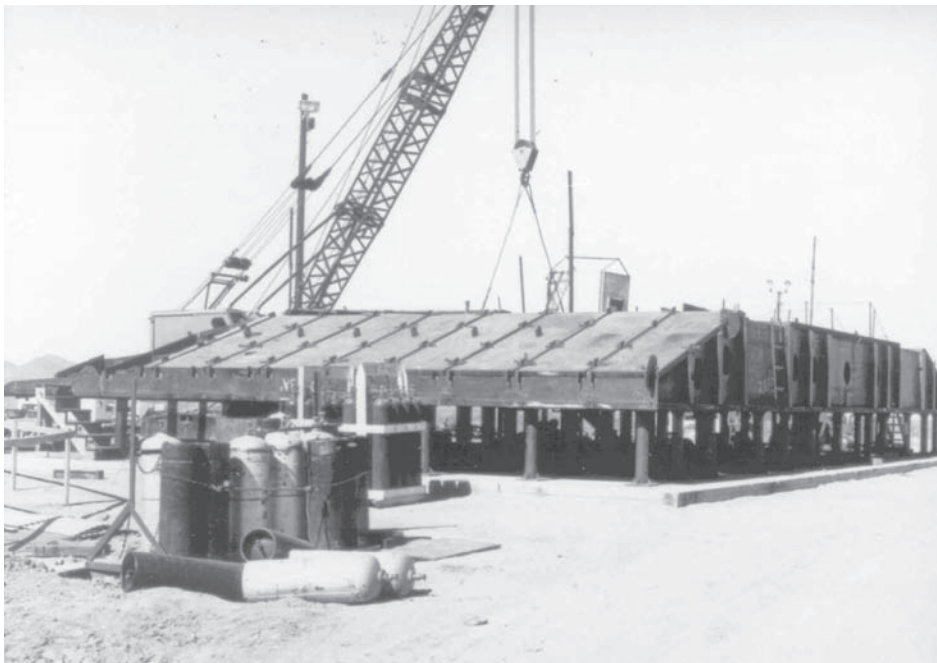
Figure 5.14b. The silo closure door sections were mounted on pedestals at the site, then welded together; the door was lowered by jacks onto temporary rail tracks for movement to the permanent tracks near the door. Courtesy of the Titan Missile Museum National Historic Landmark Archives, Sahuarita, Arizona.
