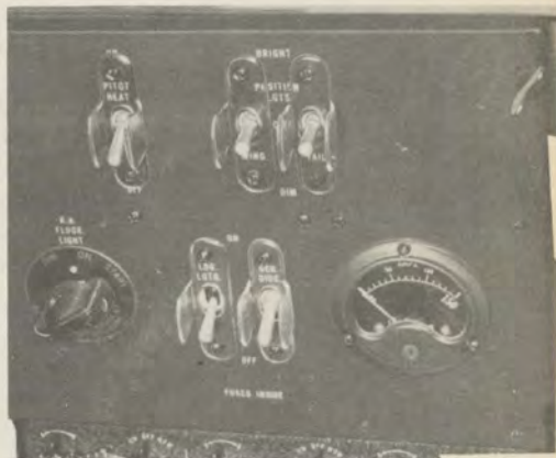
Fig. 24 RIGHT-HAND SWITCH PANEL
