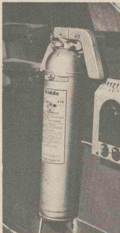
CO 2 type extinguisher located in aft pressurized compartment, aft of auxiliary equipment panel.
