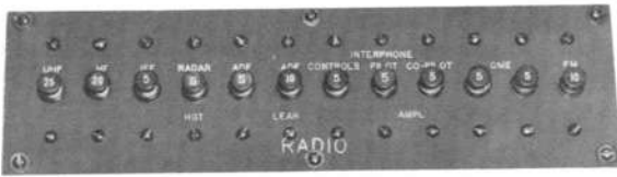
RADIO CIRCUIT BREAKER PANEL
