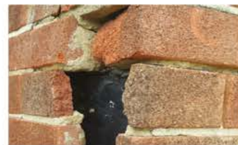
Concrete Frame Building Defects
