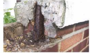
Balustrade Wall Issues
