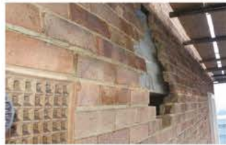
Failing Brick Slips
