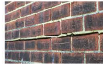
Cavity Wall Ties Failing
