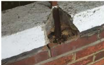
Embedded Steel Corrosion
