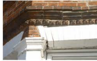
Brick Arch Failing
